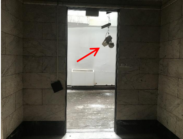
Figure 78. Damage exit sign and emergency light
