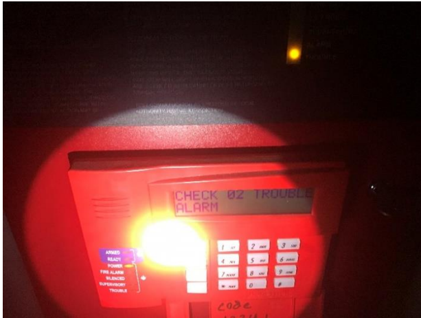
Figure 80. Fire alarm control panel in basement boiler room indicating a trouble alarm.
