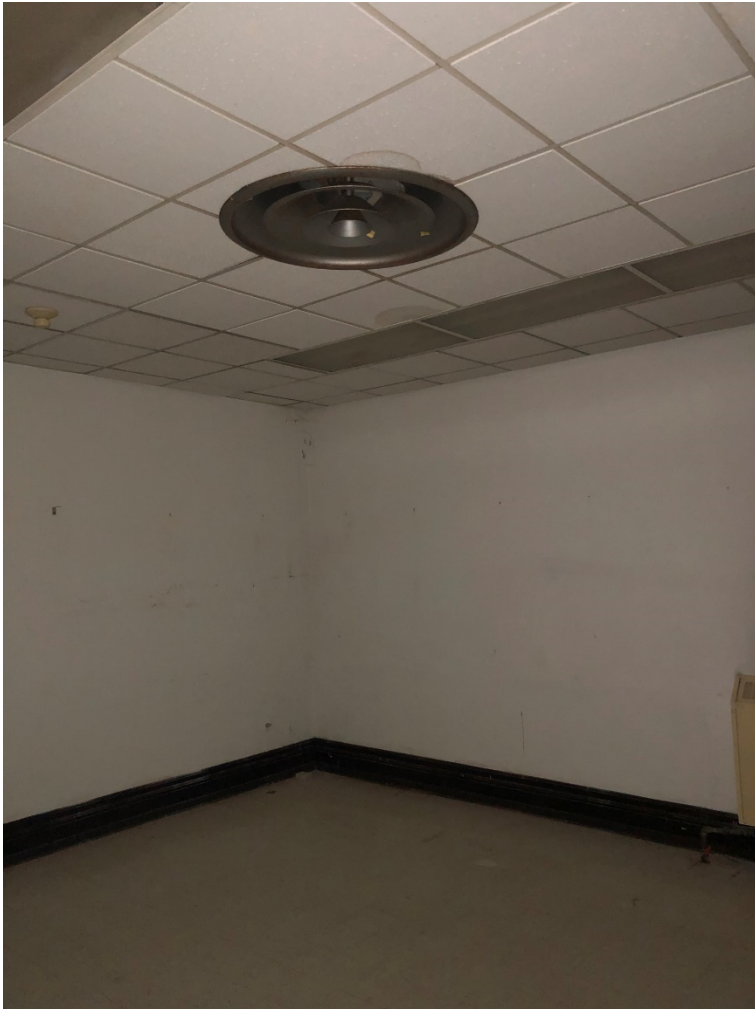
Photo OCH - 4 - 4: Office west of council chamber. Drop ceiling covering original plaster ceiling. Window openings blocked in and plastered.
