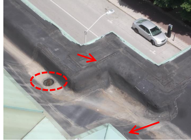
Figure 48. Un-adhered patches and missing strainer near southeast roof drain.
