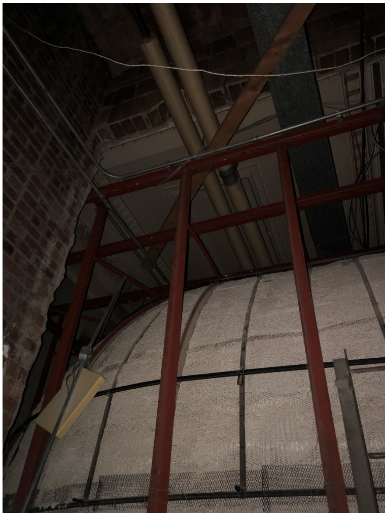
Photo OCH - 2 - 6: Behind exhibit plaster walls installed in room south of the south lobby. Typical condition found in rooms previously used for museum exhibit space.
