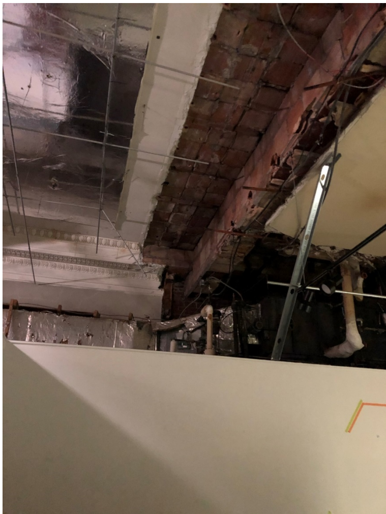
Photo OCH - 1 - 16: Room south of the south lobby. Example of plaster ceiling damage. Same room as photo OCH-1-15.
