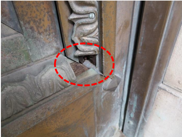
Figure 37. Open joint in bronze sheet metal with exposed and deteriorated wood core visible behind.
