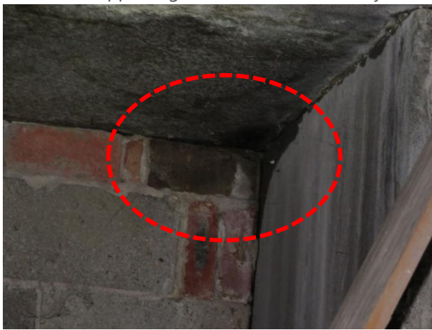
Figure 58. Water infiltration at northeast corner of vaulted sidewalk
