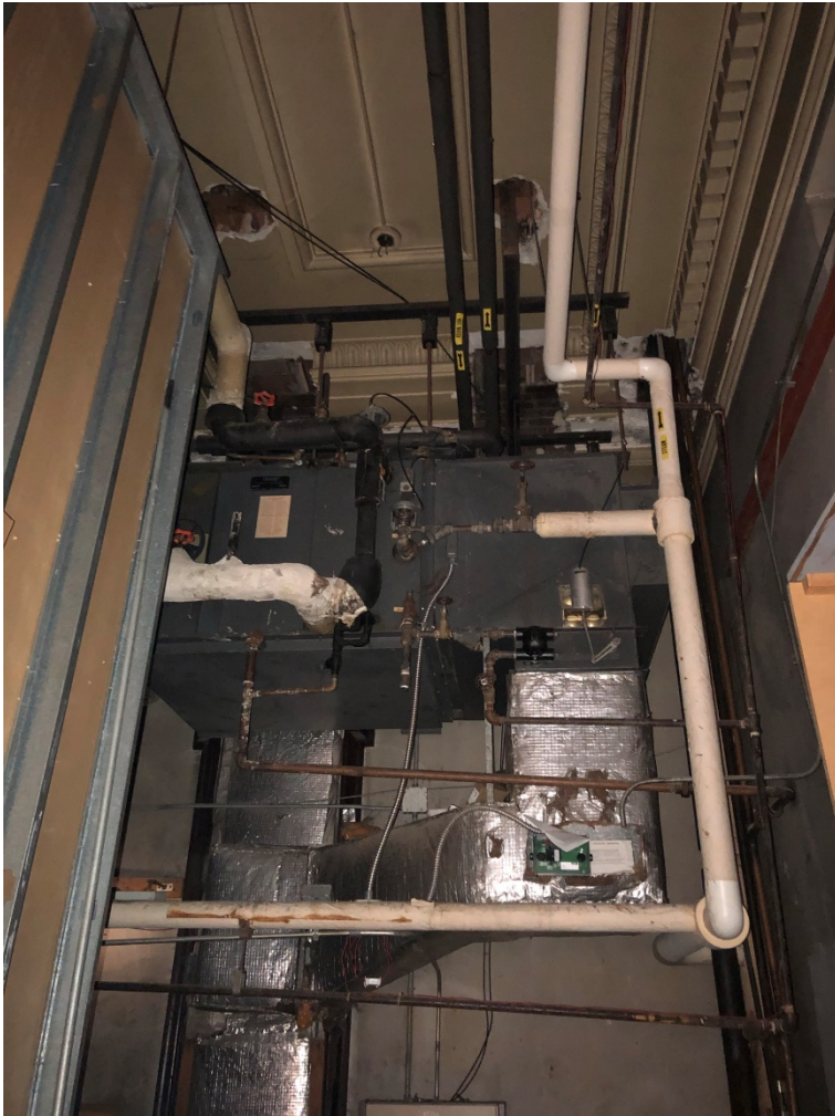
Photo OCH - 2 - 10: West end of room south of south lobby. Mechanical space located behind plaster exhibit walls. Equipment in southwest corner. Same space as photos OCH-2-8 and OCH-2-9.
