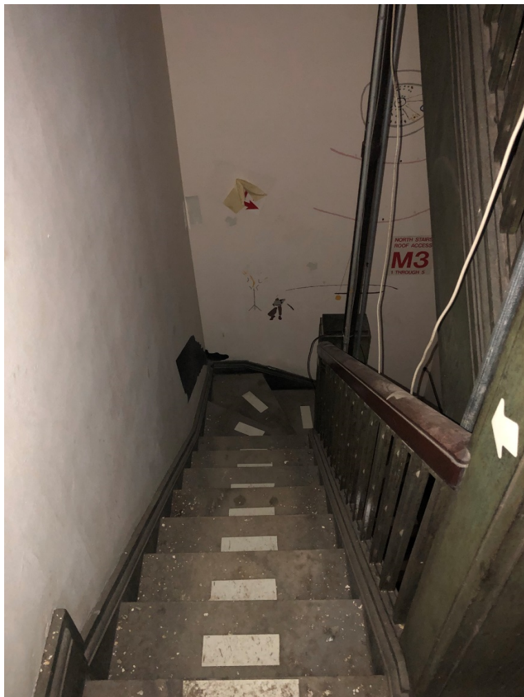
Photo OCH - 4 - 17: North private stair view from 4 th floor. Handrail only on one side.
