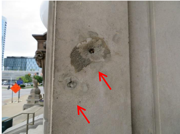
Figure 29. Spall and incipient spall at two abandoned anchors near east entrance doors.
