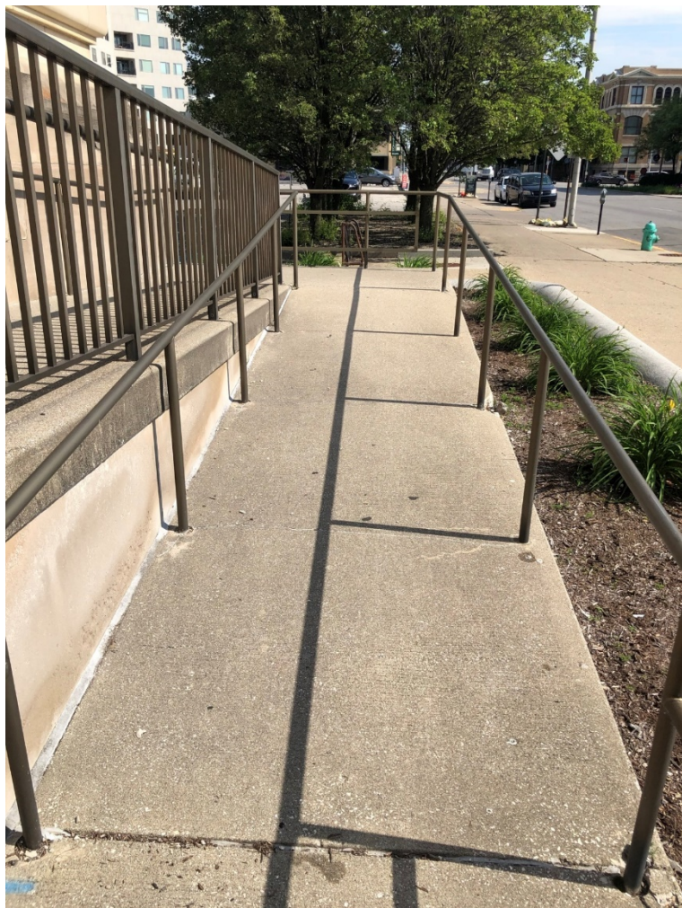
Photo OCH - EXT - 2: Ramp from street level to landing. Curb or barrier edge missing.
