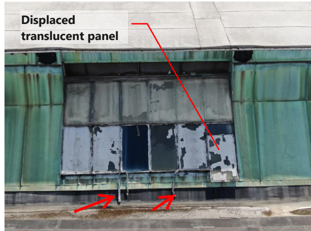
Figure 56. Deteriorated glazing at skylight along west edge of Roof Area 2.
