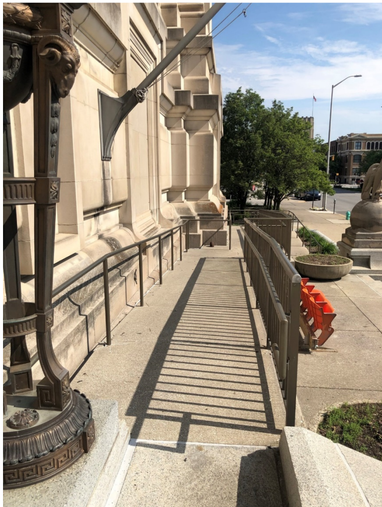
Photo OCH - EXT - 1: Ramp from building entry to landing. Curb or barrier edge protection missing.
