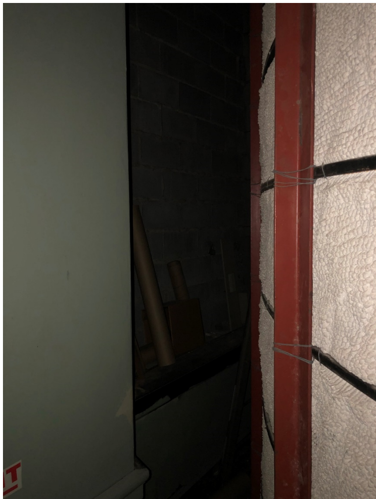
Photo OCH - 3 - 19: Behind exhibit plaster walls installed in Room north of the north lobby. Typical condition found in rooms previously used for museum exhibit space.
