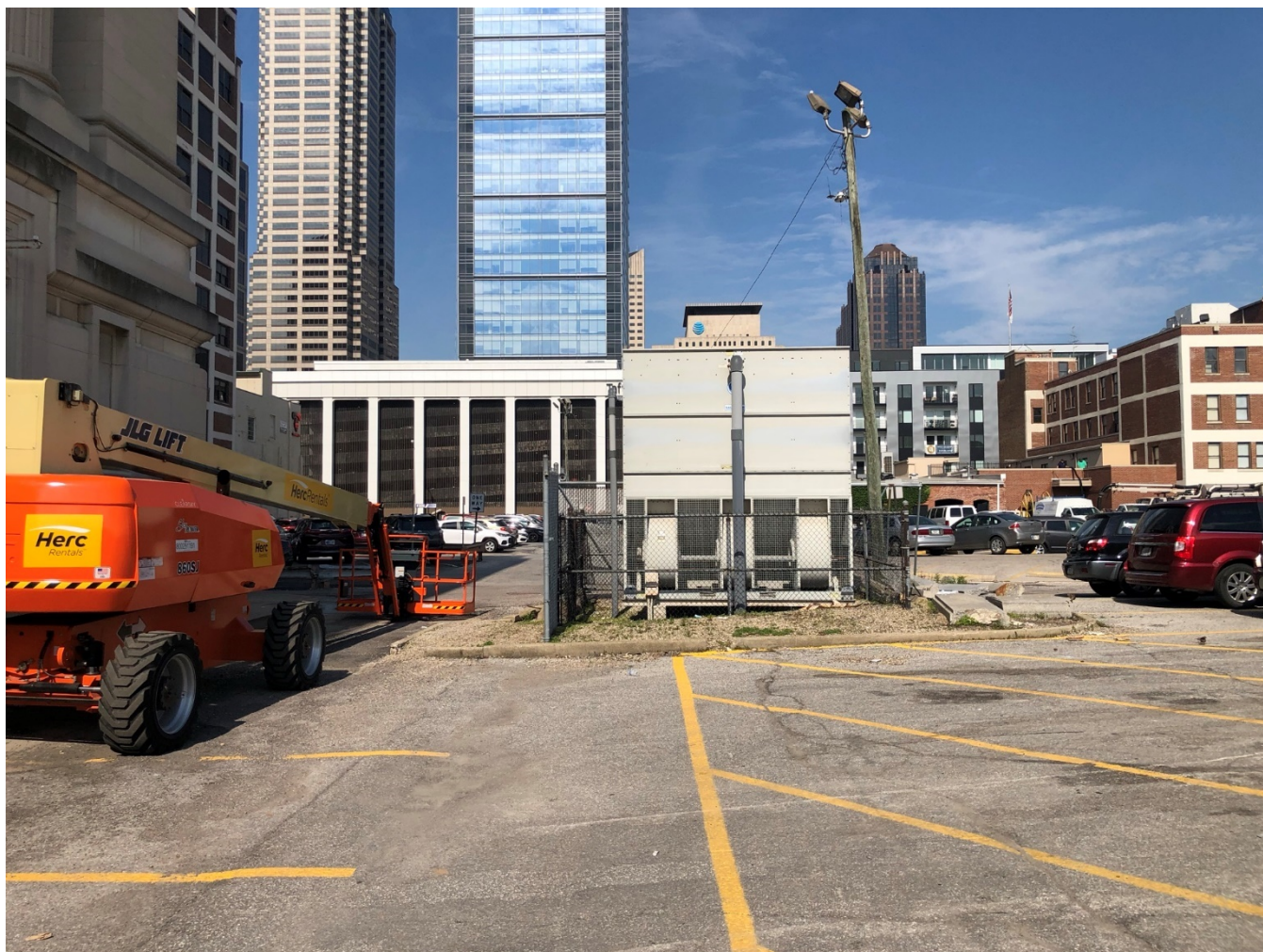
Photo OCH - EXT - 5: Cooling tower for building located in parking lot north of building.
