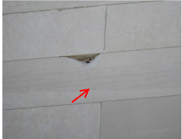
Figure 15. Spalled limestone at metal anchor showing corrosion on anchor. A crack also extends from this spall (red arrow)
