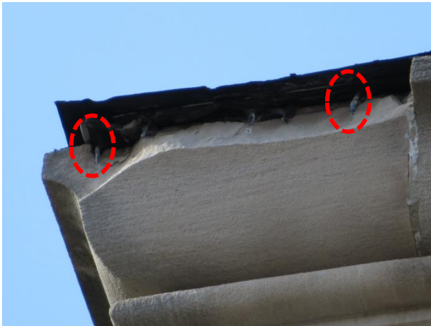
Figure 13. Wedge anchors visible at cornice spall location near northeast corner
