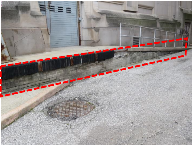
Figure 62. Cracked and missing bricks along loading dock facade.
