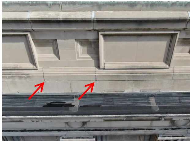
Figure 31. Displaced limestone units along south facade
