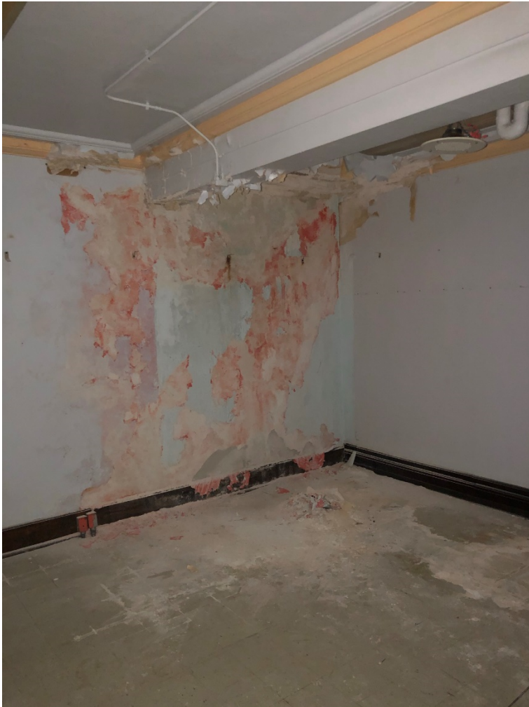
Photo OCH - 4 - 5: Office east of council chamber. Original plaster ceiling and wall damaged by water leaks. Window openings blocked in and plastered.
