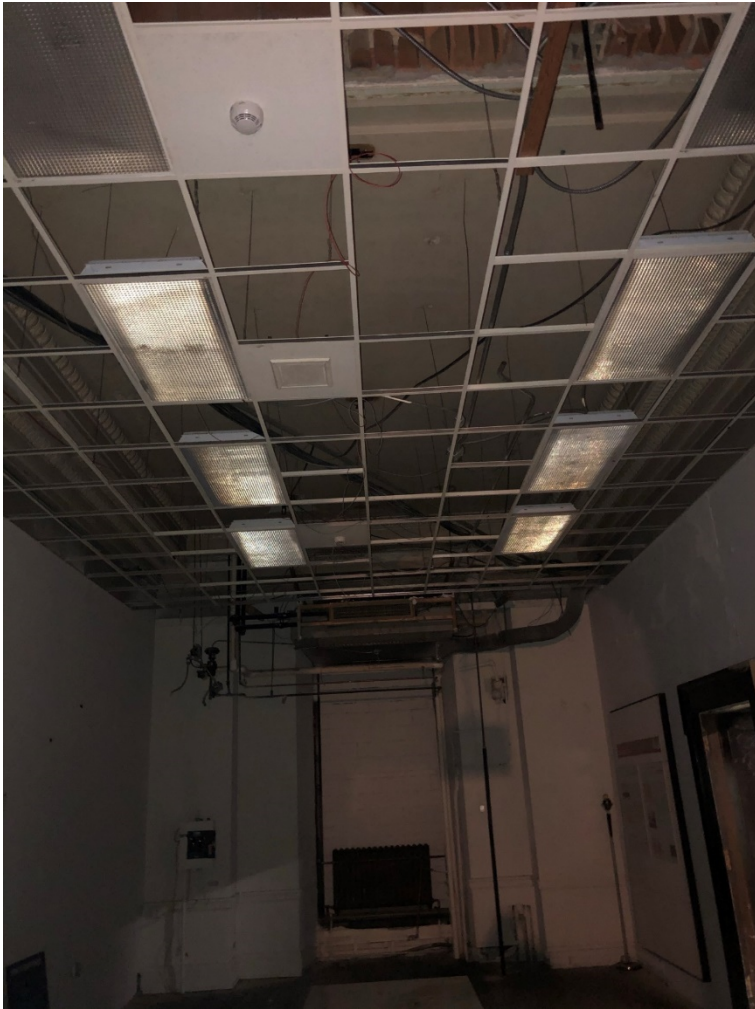
Photo OCH - 1 - 14: Room east of south lobby. Dropped ceiling covering original plaster ceiling. Original window removed and opening blocked.
