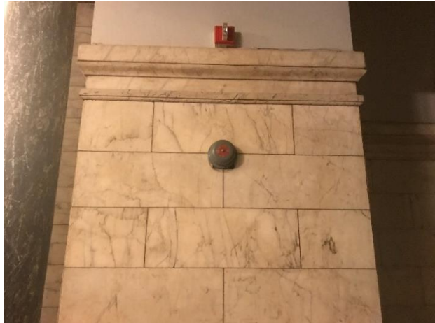
Figure 81. Strobe and alarm bell in the main atrium space
