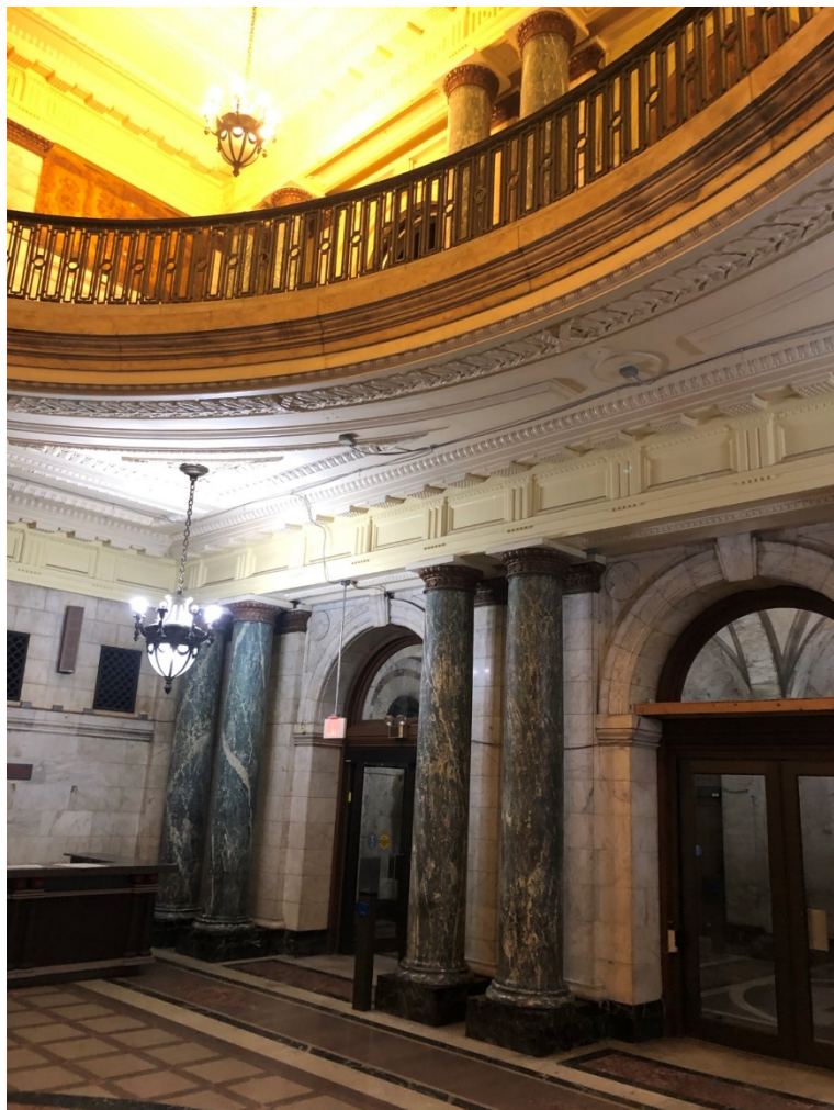
Photo OCH - 1 - 13: Rotunda viewed from south end. Electrical conduits and metal wrapped wiring surface mounted on original plaster and marble.
