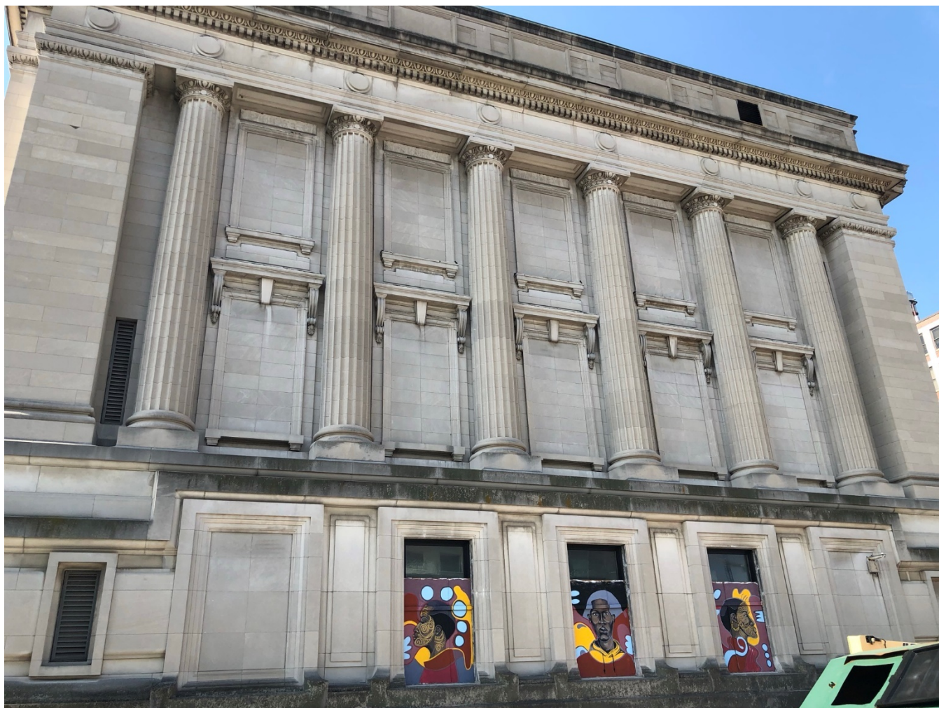
Photo OCH - EXT - 4: North elevation. Multiple original windows removed and openings blocked. Three restored windows temporarily boarded.
