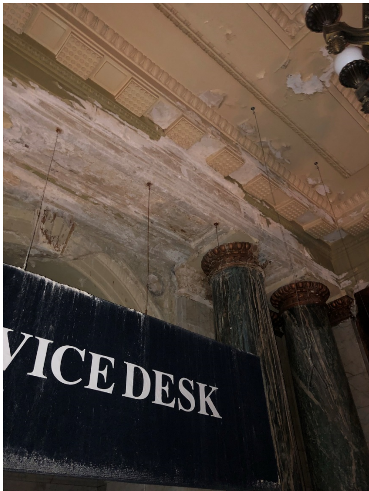
Photo OCH - 4 - 22: Southeast corner of rotunda. Original plaster ceiling and walls damaged by water leaks.
