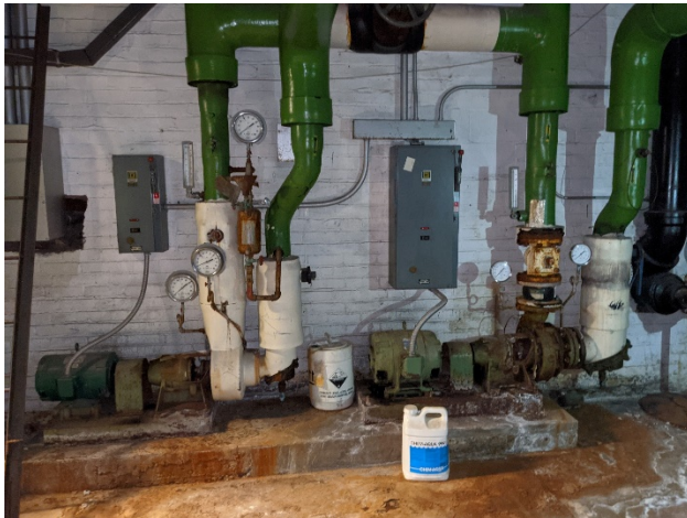
Figure 2 Chilled Water Pumps – location basement mechanical room
