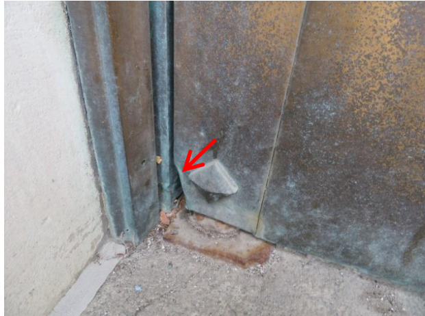
Figure 38. Dented bronze sheet metal near door hinge and surface corrosion.
