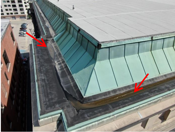
Figure 47. Ponding water along south and west portions of Roof Area 3.
