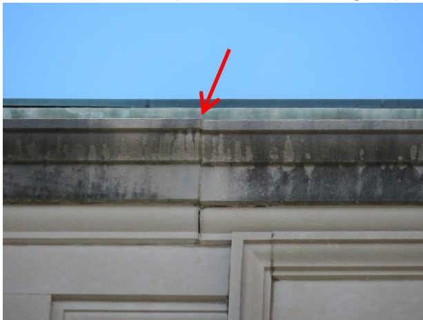
Figure 30. Displaced limestone unit at north facade.
