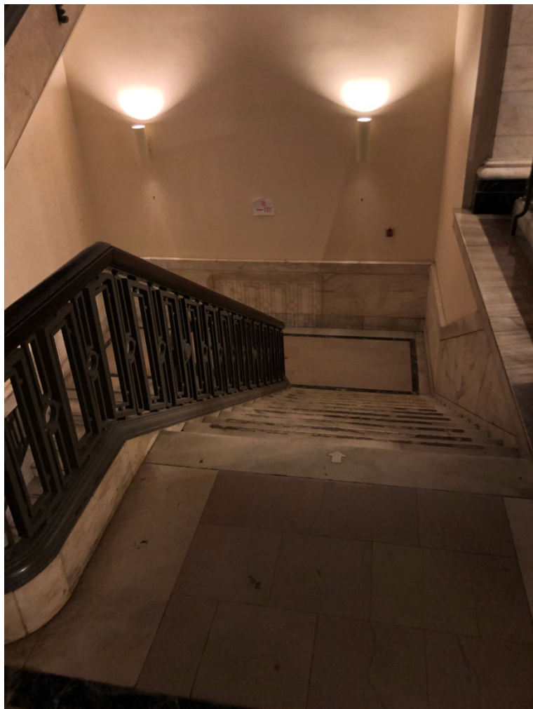
Photo OCH - 2 - 20: North side of central stairs. Handrail only on one side of stairs.
