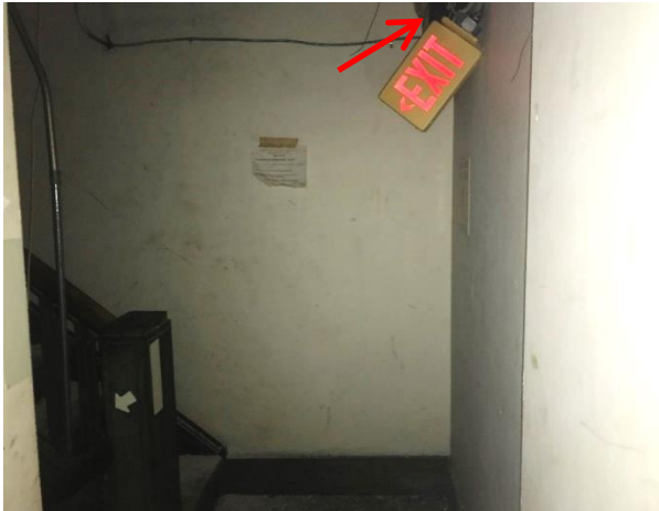
Figure 71. Penetration in stairway enclosure.
