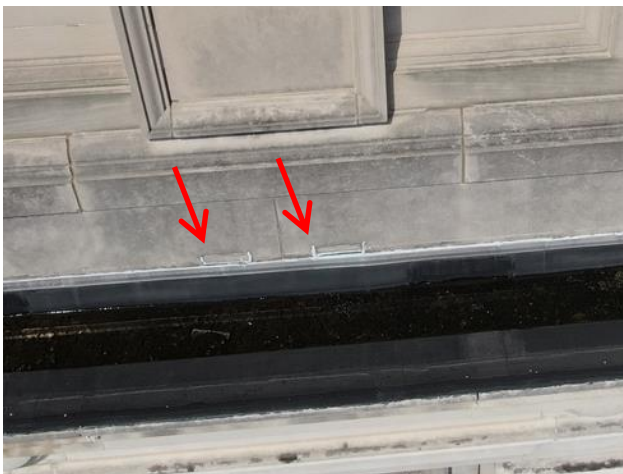
Figure 16. Two previous repairs above Roof Area 4.
