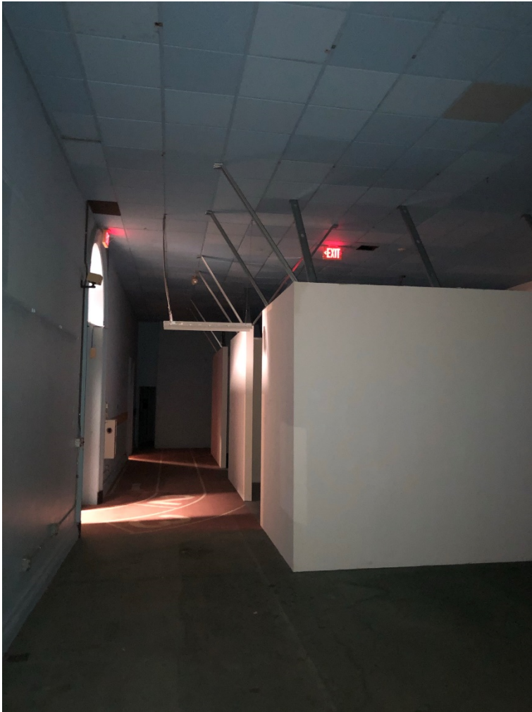
Photo OCH - 2 - 15: Room north of north lobby. Dropped ceiling coverings original plaster ceiling. Walls installed for exhibits.
