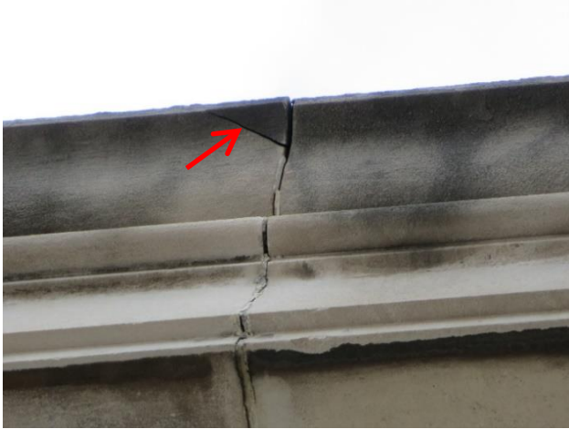
Figure 11. Incipient Spall at cornice along east facade.
