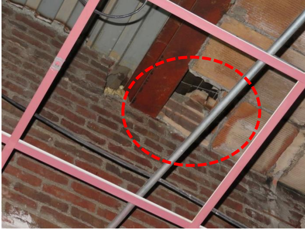
Figure 60. Missing floor tile at the corner of one flat-tile arch.
