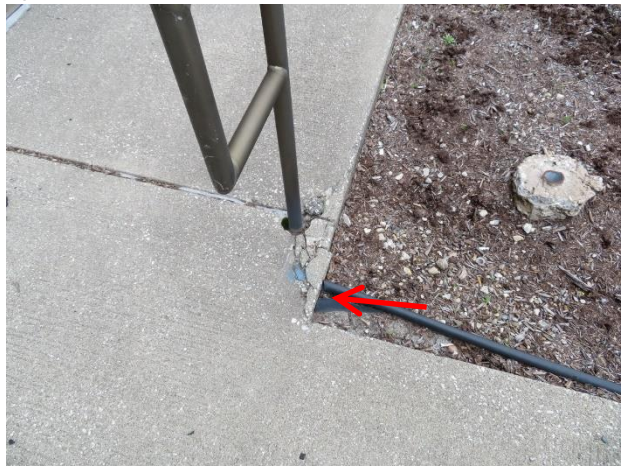
Figure 64. Cracked concrete at base of ramp handrail.
