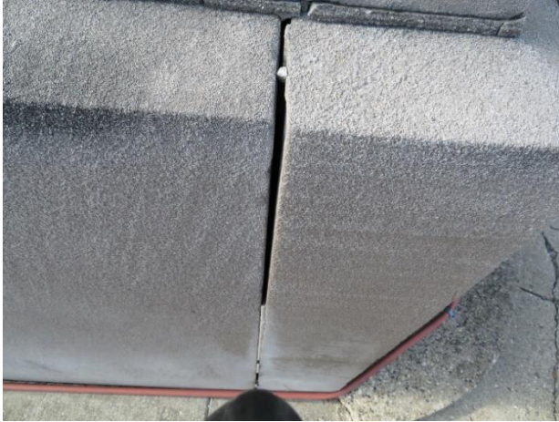
Figure 21. Open head joint at the base of north facade near northwest corner.
