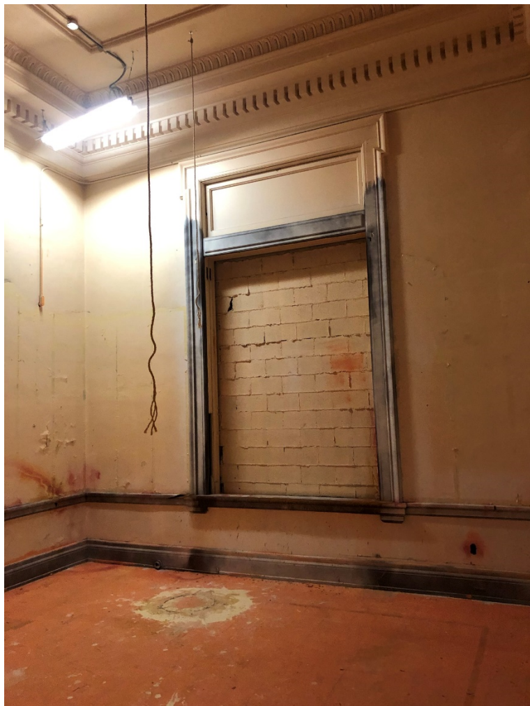
Photo OCH - 2 - 13: Room west of north lobby. Original window removed and opening blocked.
