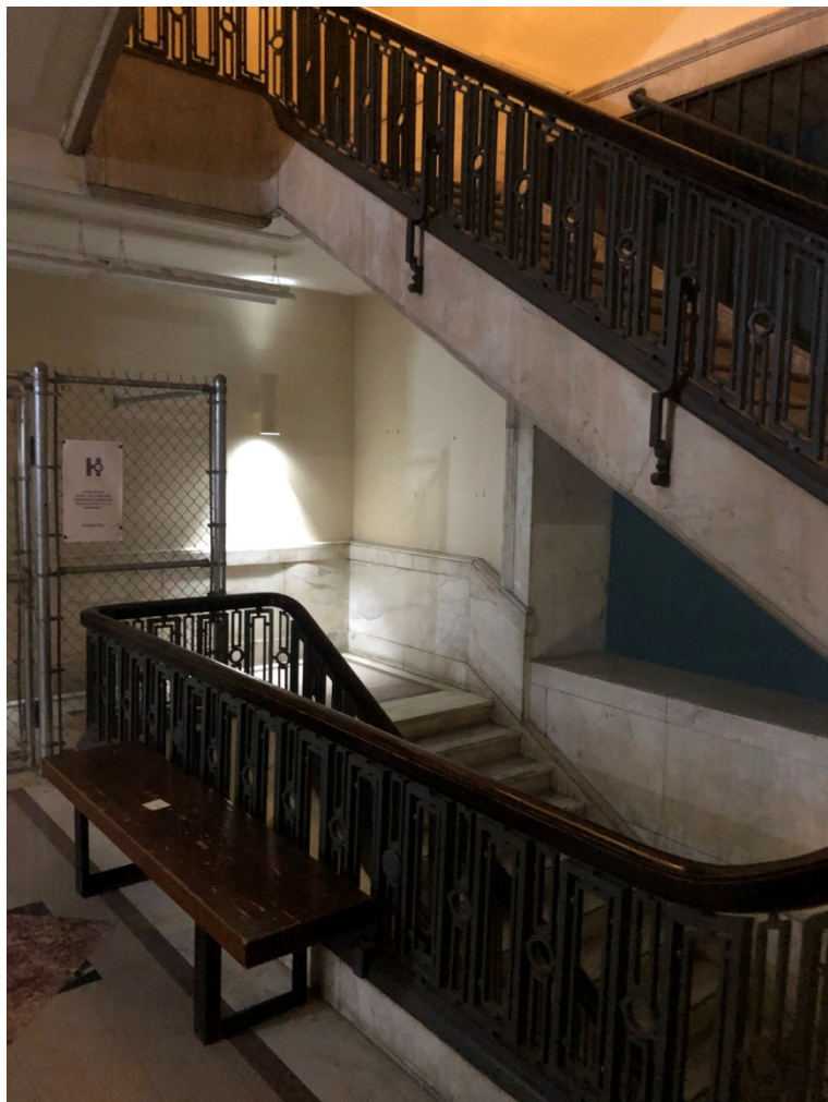
Photo OCH - 1 - 2: South side of central stairs. Chain link used to control access to basement. Handrail only on one side.
