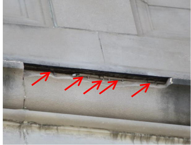
Figure 12. Spalled limestone cornice unit with metal anchors visible at fractured surface (red arrows)
