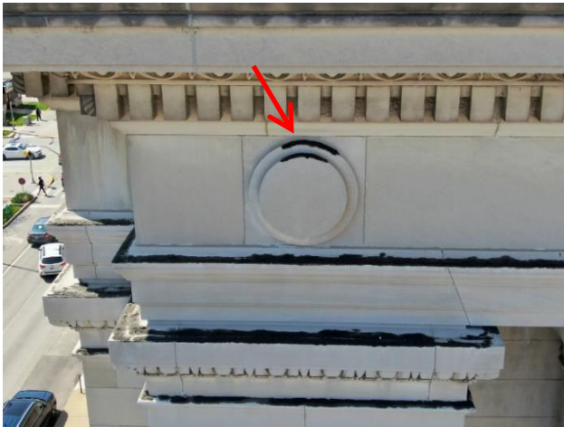
Figure 20. Unknown black material on horizontal limestone surfaces at north facade.
