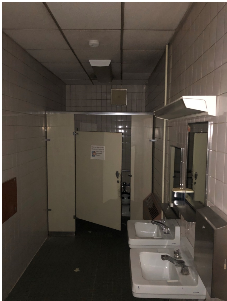
Photo OCH - 2 - 12: Bathroom south of central stairs. Because of narrow pathway, restroom will not meet accessibility requirements.
