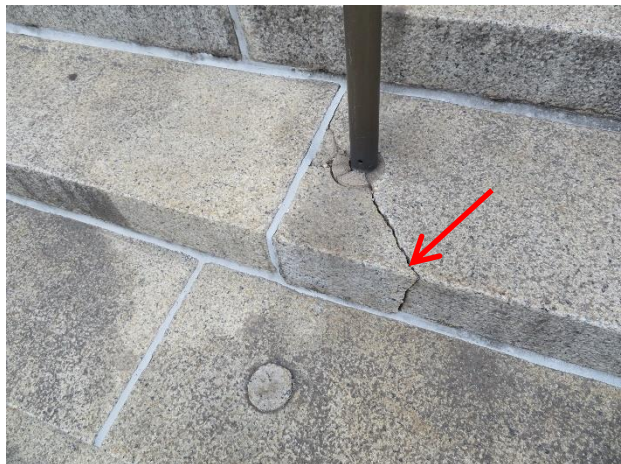
Figure 68. Corner crack at granite step near handrail post.
