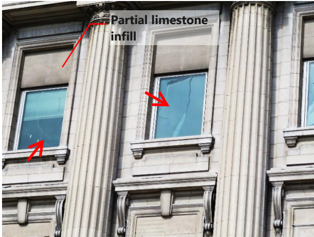
Figure 34. Broken glass at two windows along east facade.
