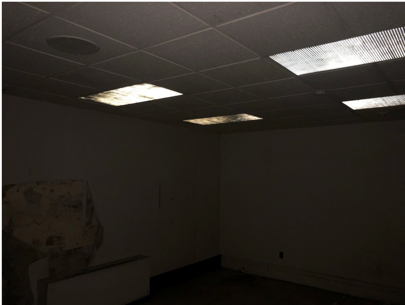
Photo OCH - 4 - 1: Office south of central stairs. Drop ceiling covering original plaster ceiling.
