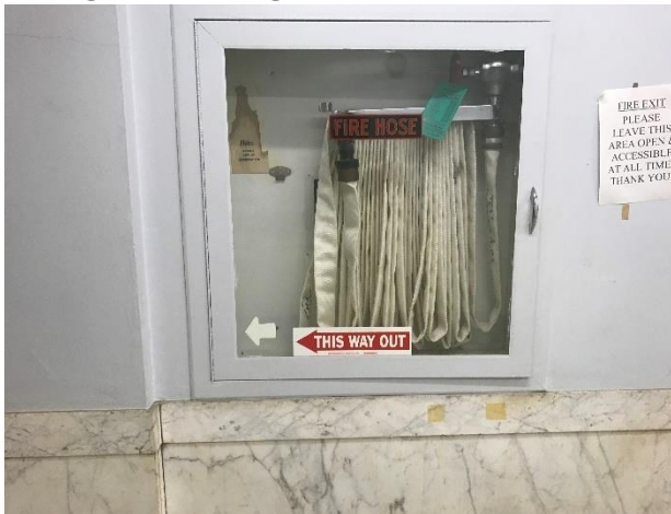
Figure 82. Fire hose cabinet with fire department connection
