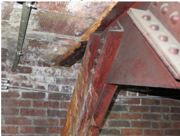
Figure 57. Surface corrosion on the top chord and diagonal bracing of roof truss.
