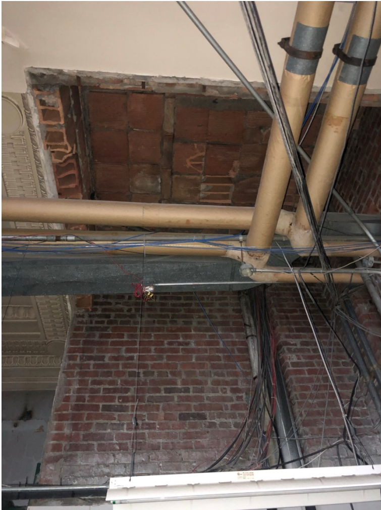
Photo OCH - 1 - 9: East end of the room north of the north lobby. Example of plaster ceiling damage. Same room as photos OCH-1-7 and OCH-1-8.
