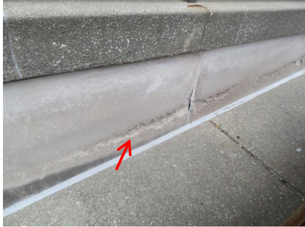
Figure 19. Deterioration of limestone units at the entrance ramp.
