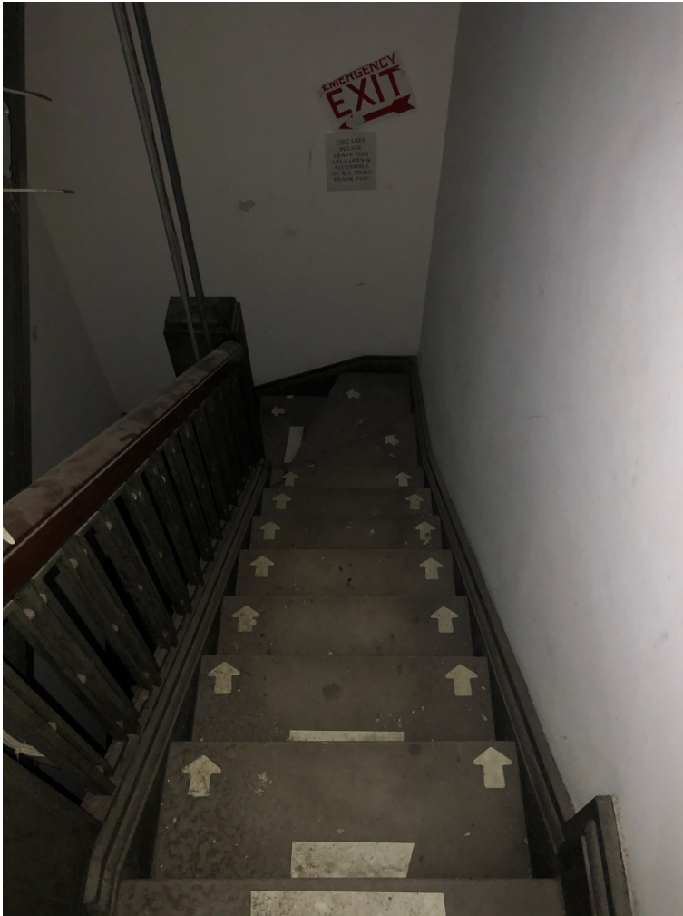
Photo OCH - 4 - 20: South private stair view from 4 th floor. Handrail only on one side.
