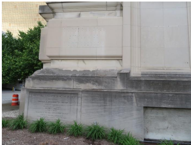
Figure 27. Atmospheric staining near base of wall.
