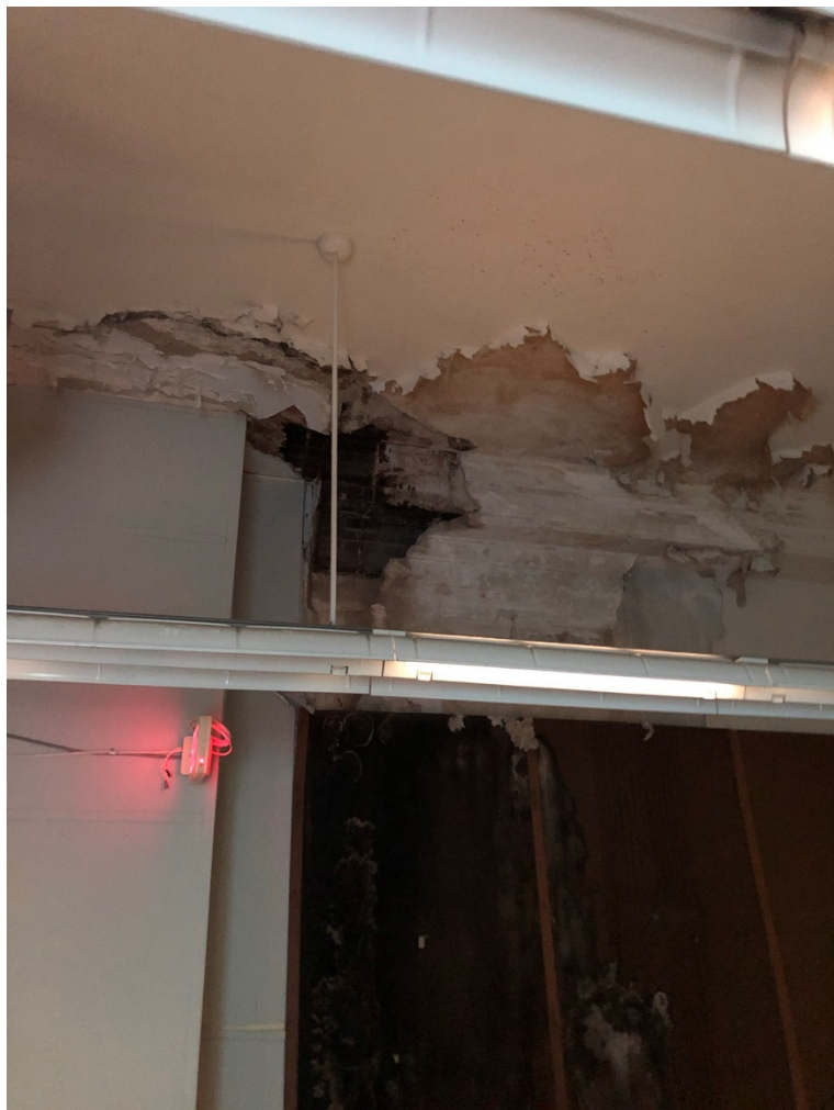
Photo OCH - 4 - 16: Office in east of north lobby. Original plaster ceiling and walls damaged by water leaks. Windows openings blocked in and plastered. Same room as OCH-4-15.
