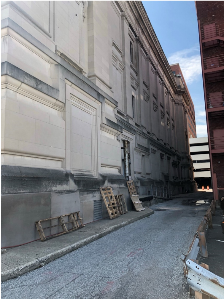
Photo OCH - EXT - 6: West elevation. Multiple original windows removed and openings blocked. Adjacent to alley.
