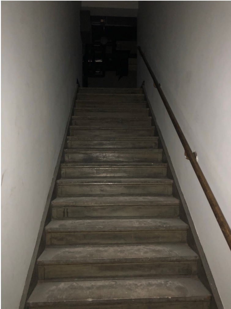
Photo OCH - 4 - 23: East stairs to mezzanine overlooking council chambers. Handrail only on one side.
