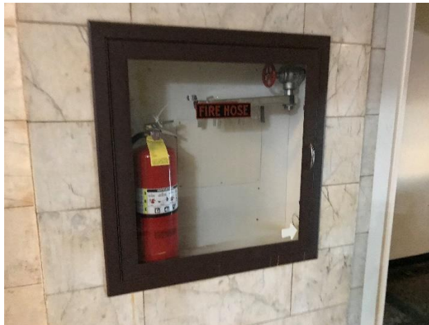
Figure 83. Fire hose cabinet with hose removed and fire extinguisher located in the cabinet.
