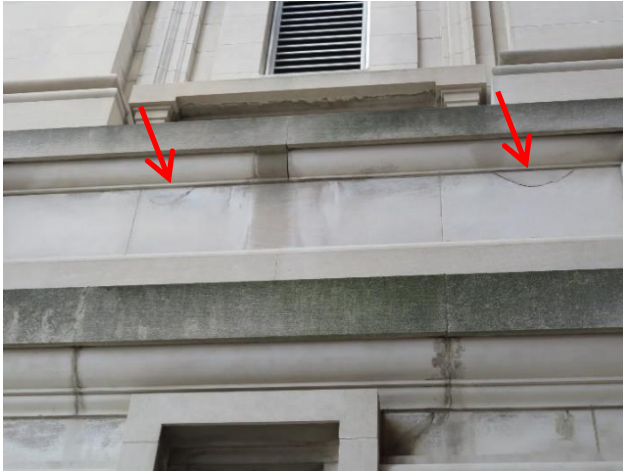
Figure 14. Two incipient limestone spalls at the west facade.
