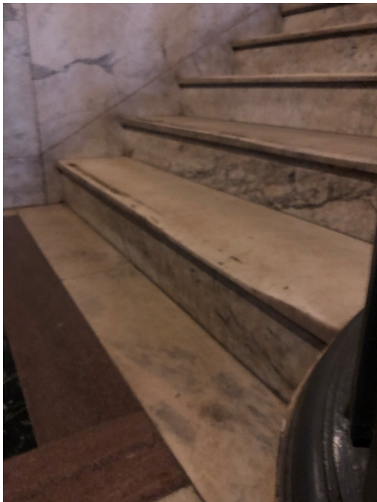
Photo OCH - 1 - 4: North side of central stairs. Stairs leading to second floor. Significant wear on stair treads.
