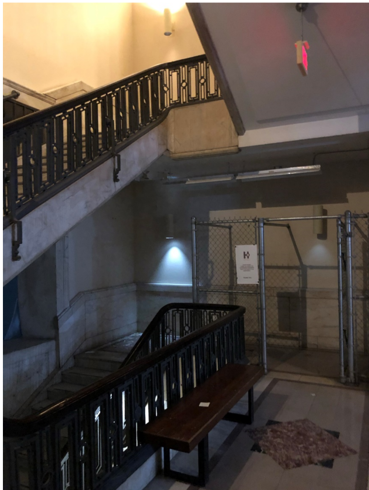
Photo OCH - 1 - 1: North side of central stairs. Chain link used to control access to basement. Handrail only on one side.
