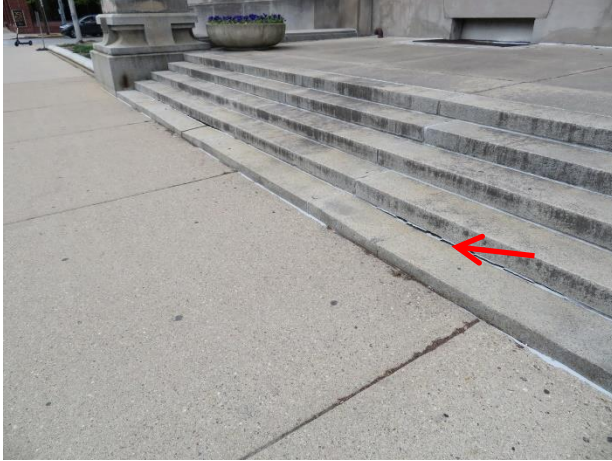
Figure 65. Deteriorated sealant at east entrance steps.
