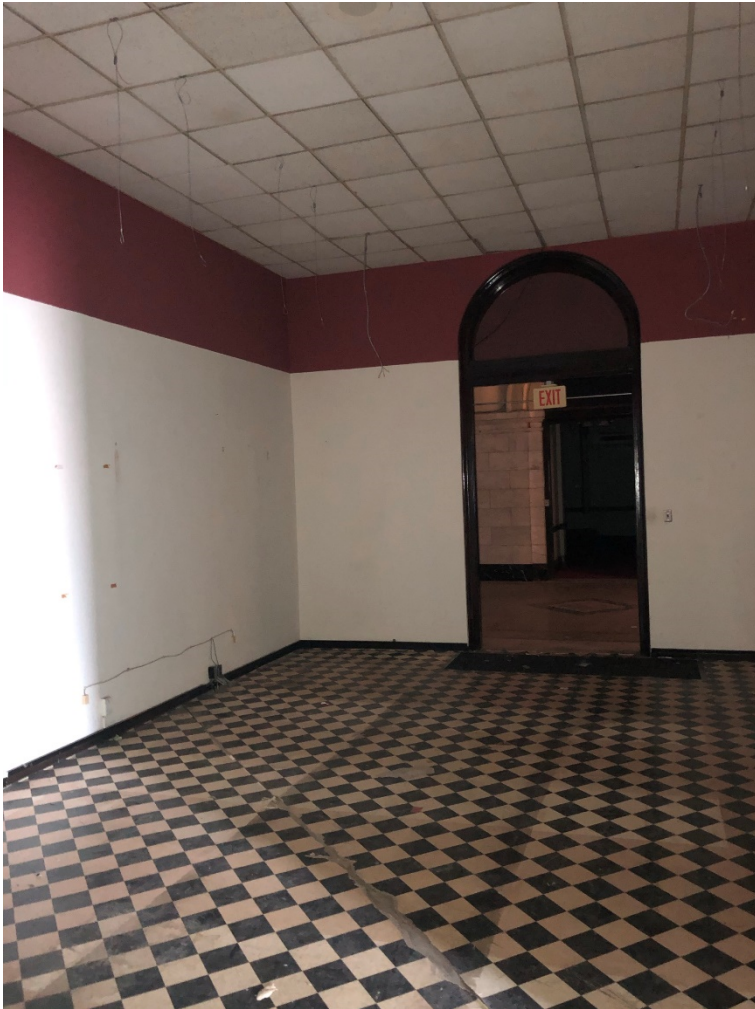
Photo OCH - 3 - 7: Room east of the south lobby. Dropped ceiling covers original plaster ceiling. Damaged floor tile. Testing for hazardous materials required.
