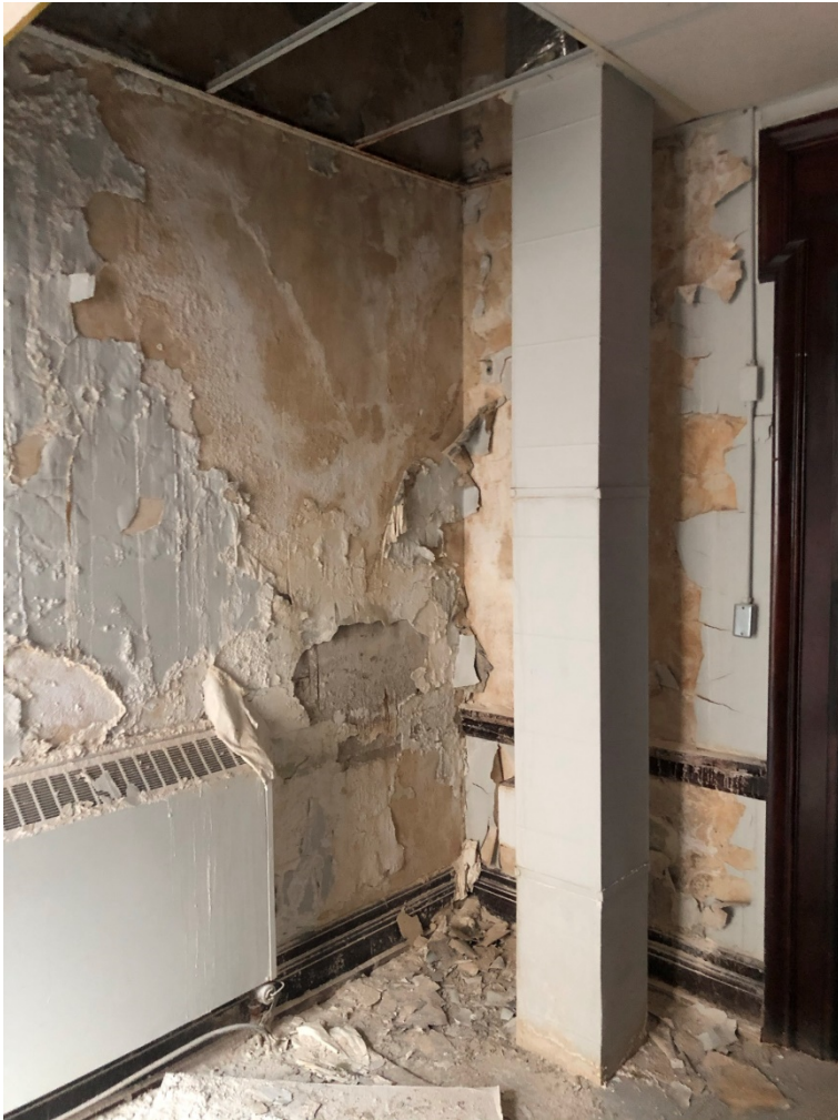
Photo OCH - 4 - 6: Office east of rotunda. Dropped ceiling covering original plaster ceiling. Original plaster ceiling and wall damaged by water leaks. Window openings blocked in and plastered. Same room as Photo OCH-4-7.
