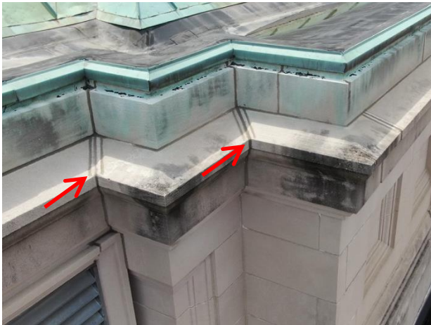
Figure 23. Upward facing sealant joints near the north re-entrant corner on the west facade.
