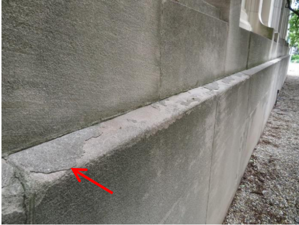
Figure 18. Deterioration of horizontal limestone surface on south facade.
