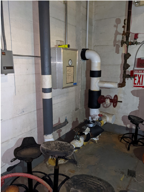
Figure 5 Domestic Water Service – location basement east wall
