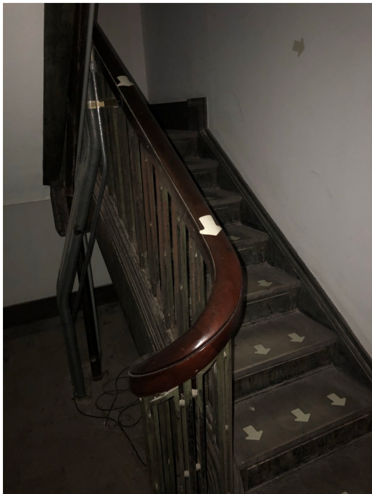
Photo OCH - 1 - 11: Bottom of north private stairs. Handrails only on one side. Stairs do not exit to the exterior or to an egress path.
