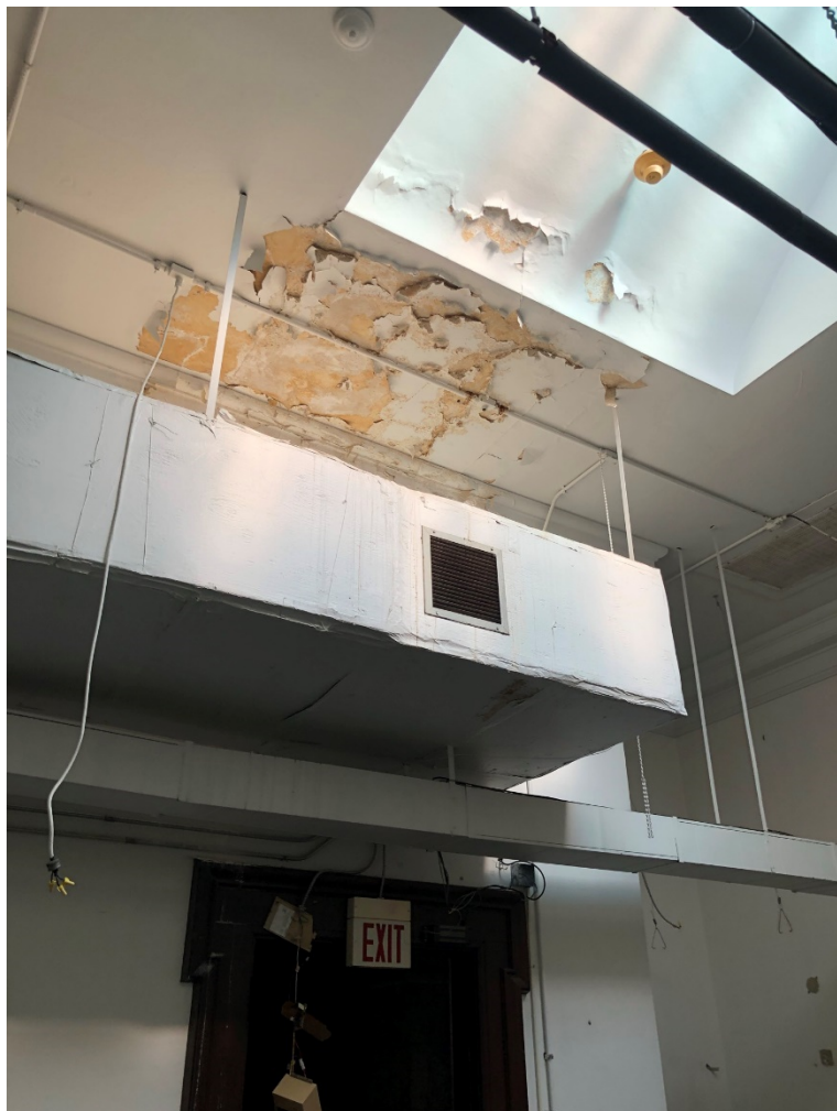
Photo OCH - 4 - 8: Office east of rotunda. Original plaster ceiling and wall damaged by water leaks. Window openings blocked in and plastered. Same room as Photo OCH-4-9.
