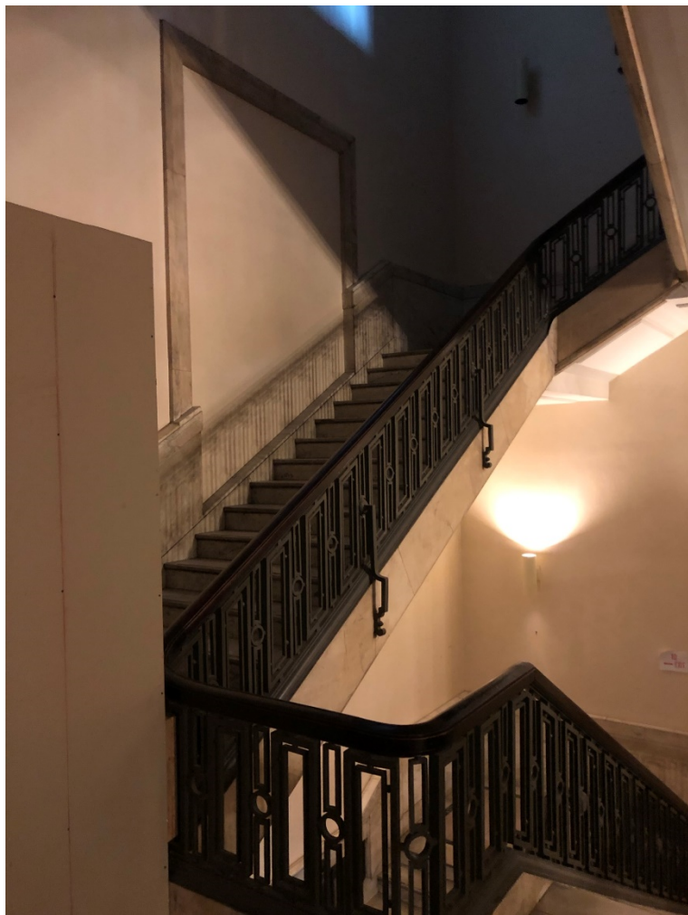
Photo OCH - 2 - 19: North side of central stairs. Wall and door installed to control access above second floor. Original windows removed and openings blocked. Handrail only on one side of stairs.
