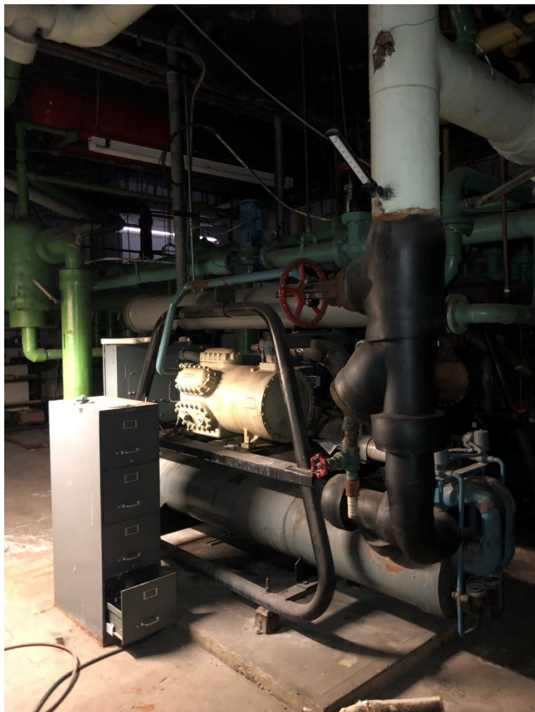
Photo OCH - B - 13: Mechanical room in northwest corner of basement.
