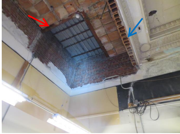
Figure 61. Metal deck visible at area of removed flat-tile arch sub-floor (red arrow). Also note unsupported clay tiles (blue arrow). These appear to be remnants of an original interior partition wall, subsequently partially demolished.
