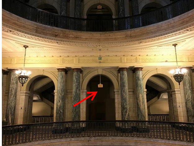
Figure 79. Burnt out exit signage in main atrium space
