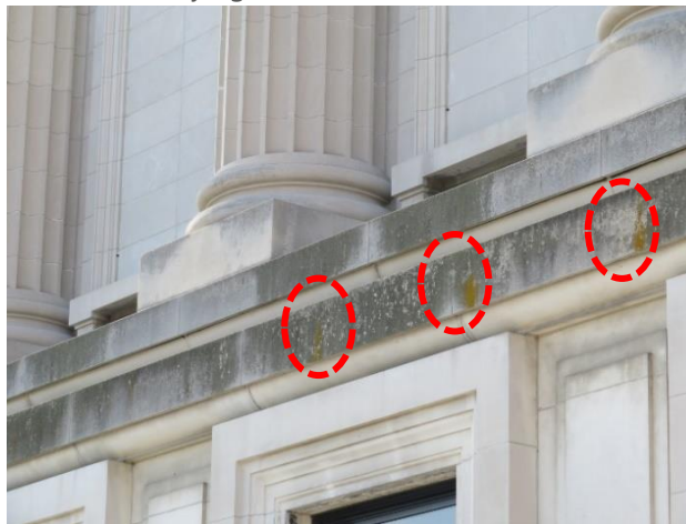
Figure 26. Atmospheric staining on vertical surface of north facade. Biological growth within stained areas is shown by red dashed ellipses.
