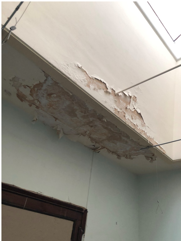
Photo OCH - 4 - 11: Lobby north of rotunda. Original plaster ceiling and walls damaged by water leaks. Same room as Photo-OCH-4-11.
