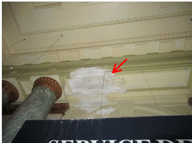
Figure 40. Water damage near the eastern edge of the atrium at the fourth floor.
