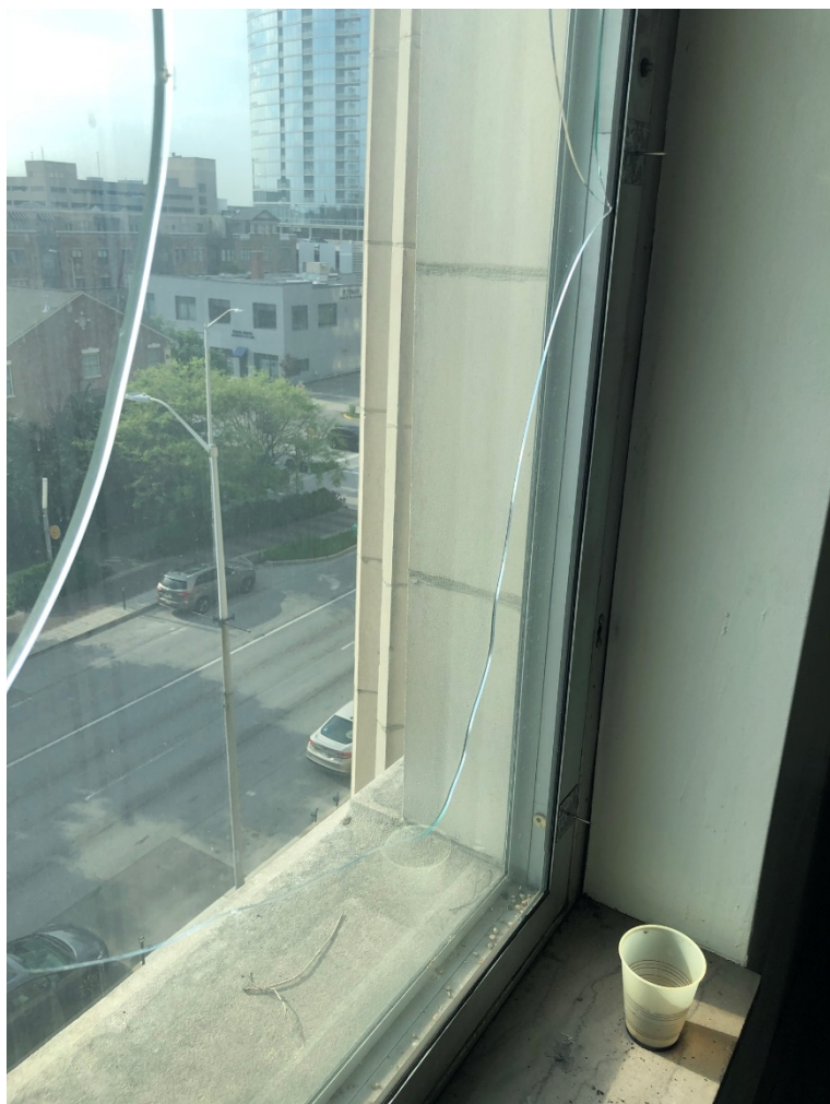
Photo OCH - 3 - 3: Exterior window in room east of rotunda. Exterior pane broken. Same room as Photos OCH-3-4 through OCH-3-6.
