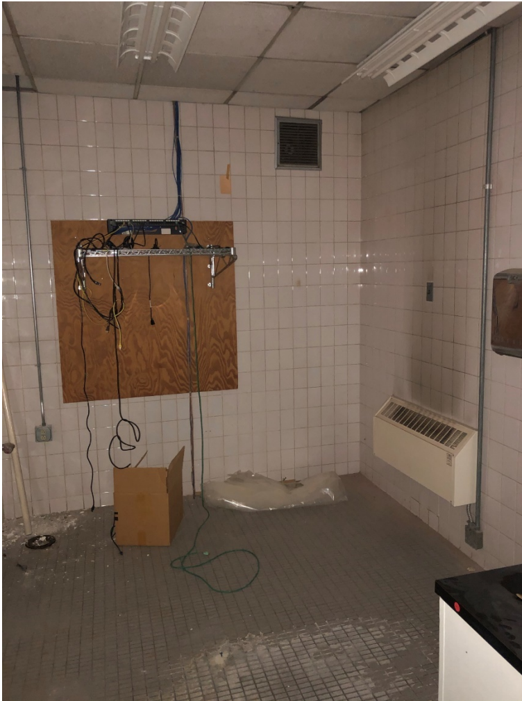
Photo OCH - 4 - 2: Former bathroom east of council chamber utilized as MDF room.
