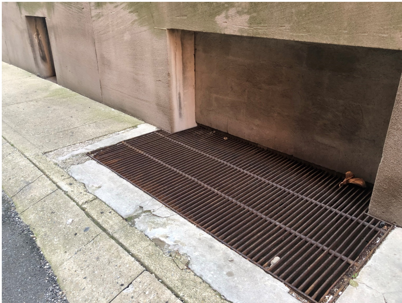
Photo OCH - EXT - 10: West elevation. Window wells at basement window openings. Window openings blocked.
