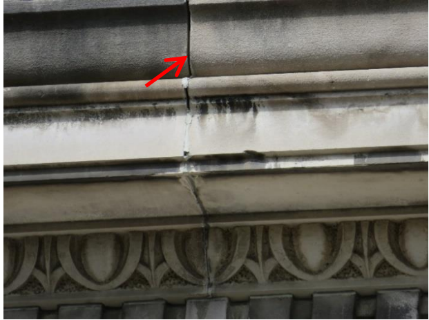
Figure 22. Open head joint below cornice along east facade.
