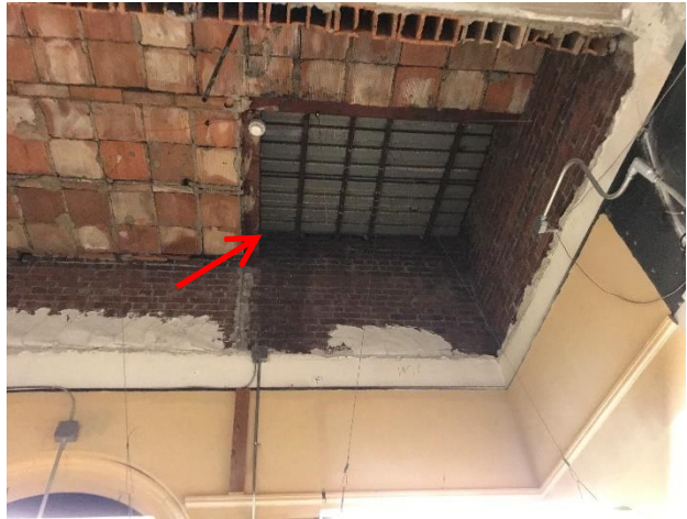
Figure 75. Damaged structural fireproofing near the freight elevator on the first floor.
