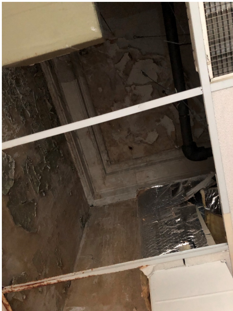
Photo OCH - 4 - 7: Office east of rotunda. Dropped ceiling covering original plaster ceiling. Original plaster ceiling and wall damaged by water leaks. Window openings blocked in and plastered. Same room as Photo OCH-4-6.
