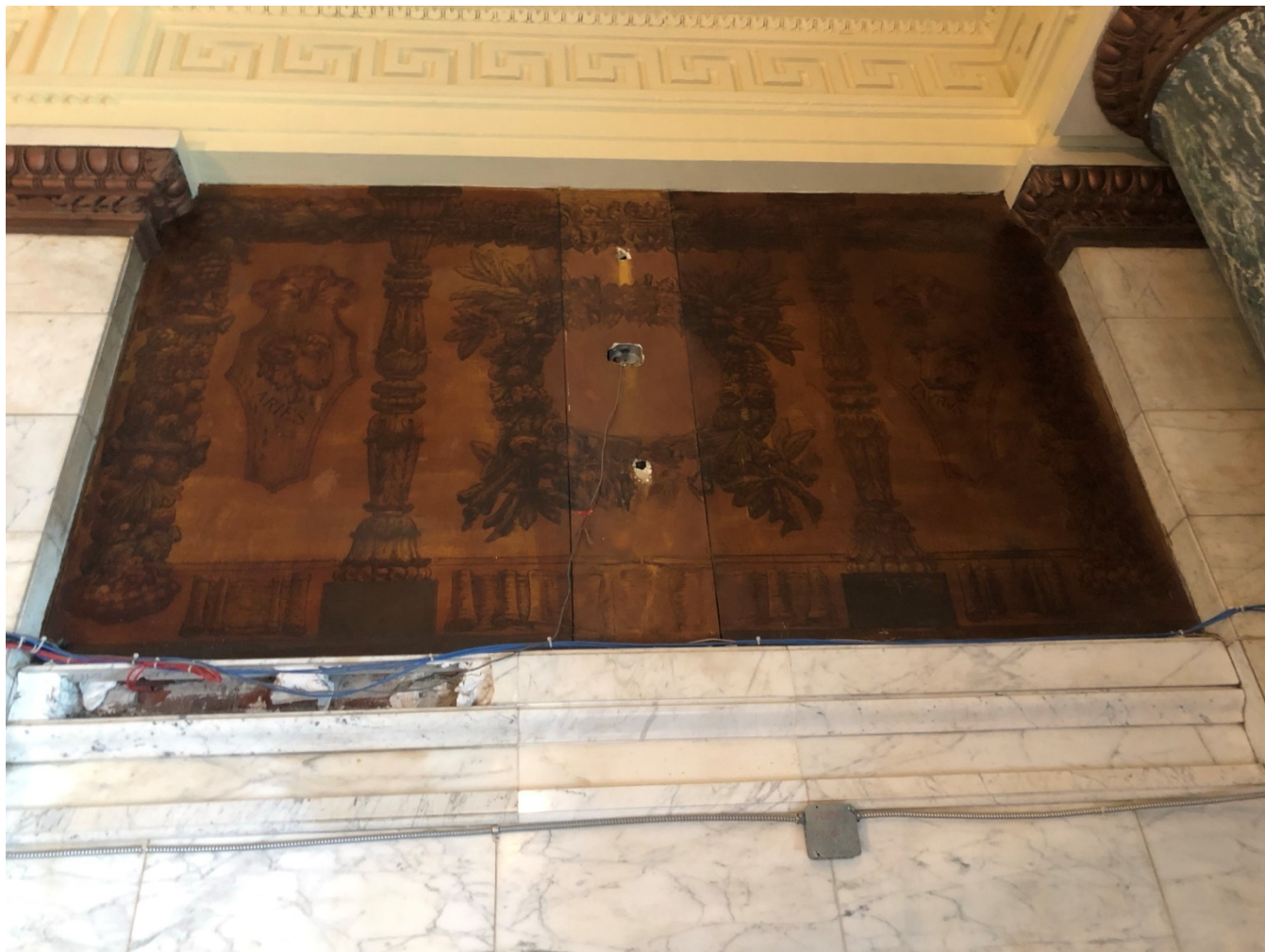
Photo OCH - 3 - 15: Northeast corner of rotunda. Damaged artwork and marblework. Utility boxes and wrapped wiring surface mounted on marblework.
