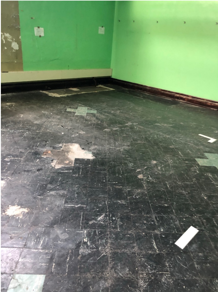
Photo OCH - 4 - 14: Office north of rotunda. Damaged floor tile. Testing for hazardous materials required. Same room as OCH-4-14.
