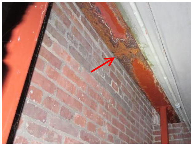
Figure 59. Surface corrosion on supplemental steel framing below vaulted sidewalk.
