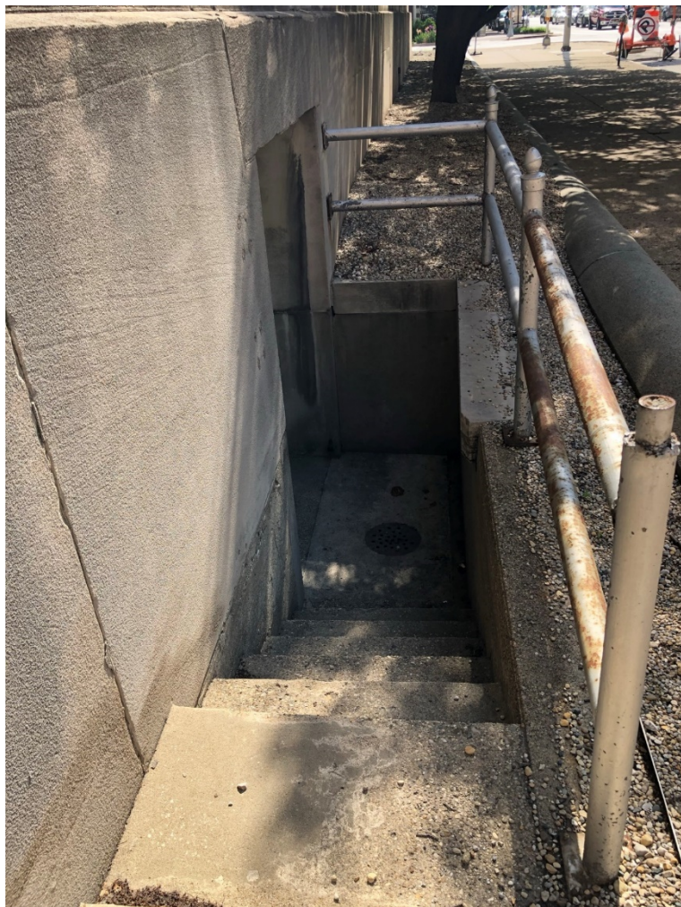
Photo OCH - EXT - 12: Stairs to basement egress on south elevation adjacent to Ohio Street. No handrails. Guardrail is not code compliant.
