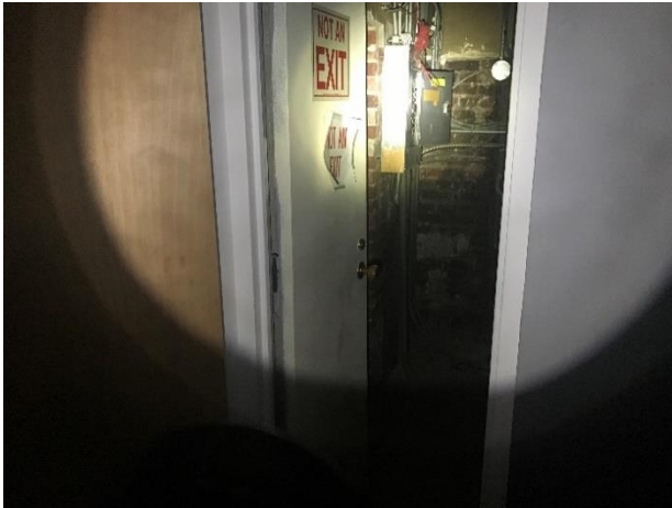
Figure 72. Typical electrical room
