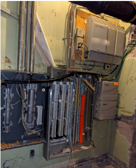
Figure 4 Existing IT Infrastructure – location basement mechanical room
