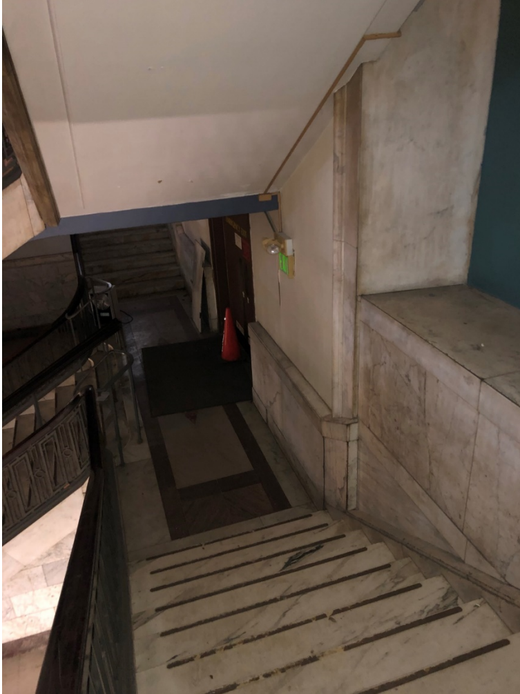
Photo OCH - B - 1: North side of central stairs leading to basement landing. Egress stairs on right. Handrail only on one side.
