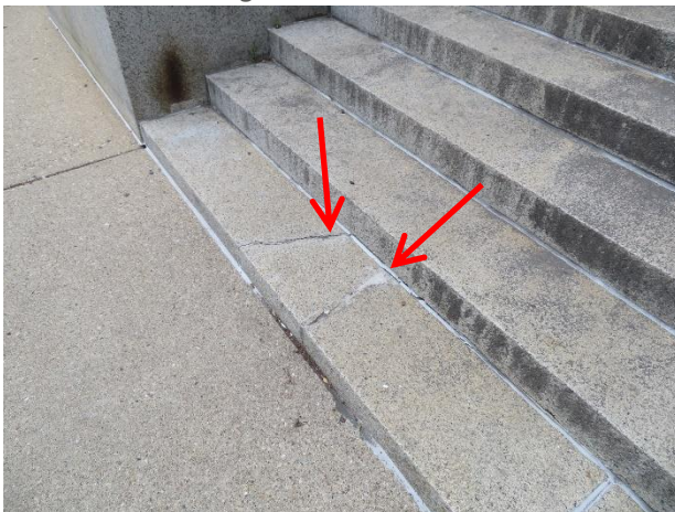
Figure 67. Cracked granite step near east entrance.
