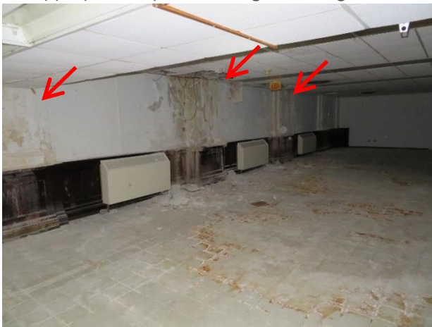
Figure 39. Water damage along the south wall at the fourth floor.
